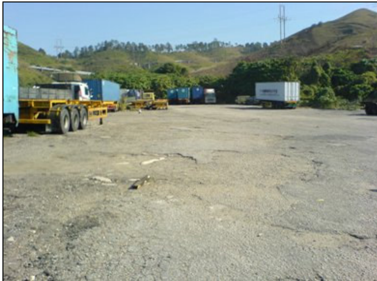
Photograph 7-1 Existing Poor Condition of the Hardstanding within the Site
